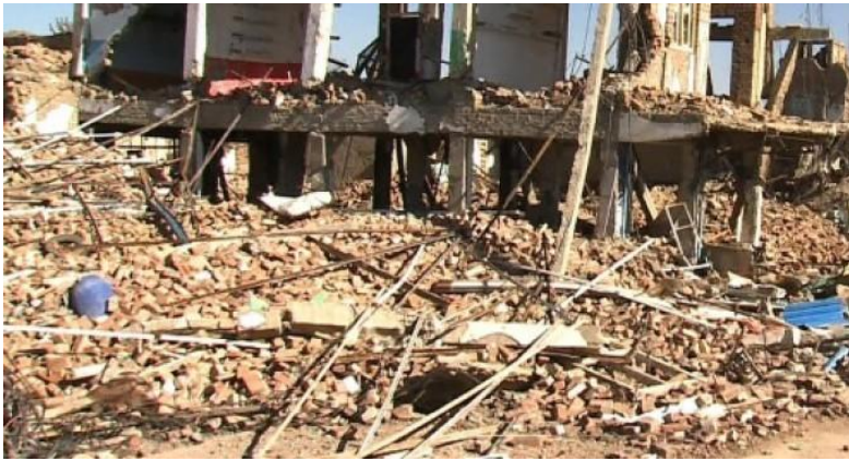
Source: Tribal News Network. (2016, May 24). Tribesmen from Miranshah Ask Government To Rebuild Their Damaged Houses. Retrieved from TNN: http://www.radiotnn.com/tribesmen-from-miranshah-ask-government-to-rebuild-their-damaged-houses/ . Accessed on February 23, 2017.
